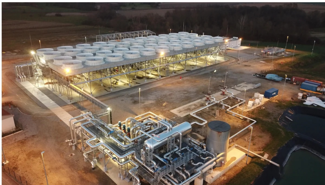
The Velika Ciglena geothermal plant in Ciglena, Croatia. (Turboden)
